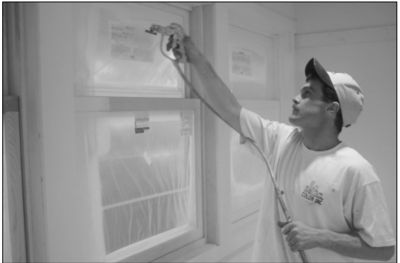
Eric Poor applies primer to the windows in President Osgood's new dining room.
